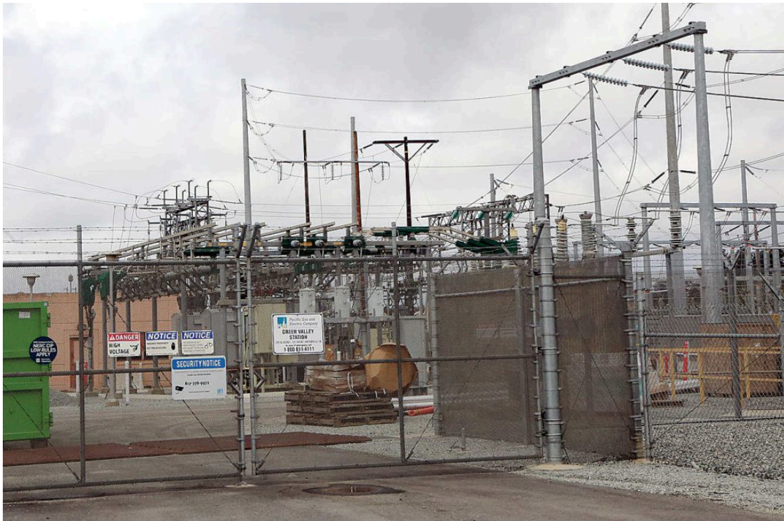
This Pacific Gas and Electric substation at the end of Minto Road in Watsonville is a proposed site for a new Battery Energy Storage System. (Tarmo Hannula/The Pajaronian)
